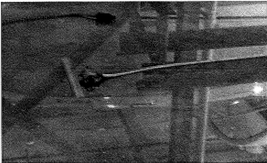
Water accumulation at the floor of the marina structure is considered at least partially due to water entry on the planter and stairwell juncture at the east facade wall of the tower.
